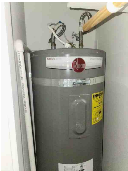
Hot Water Heater Unit B
