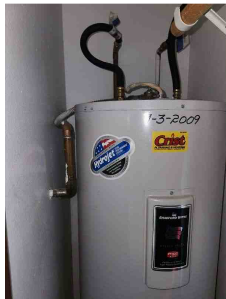
Hot Water Heater Unit A
