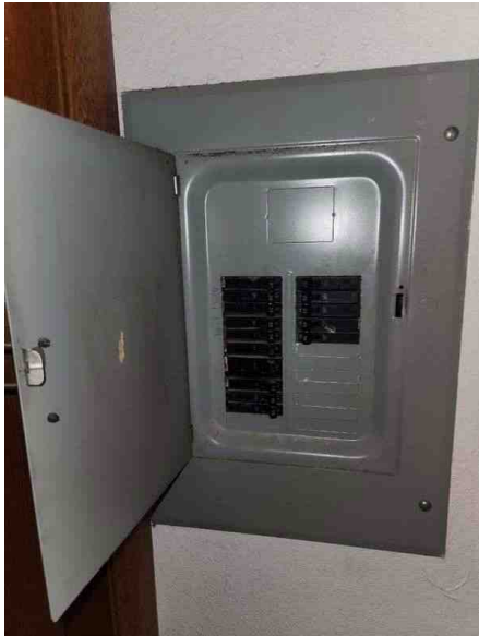
Electric Unit A
